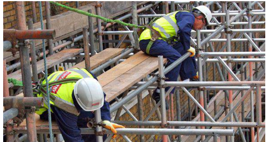
Scaffolding is a large part of the cost for replacing glazing. By including window upgrades as part of routine maintenance and upgrade work, costs can be minimized.
